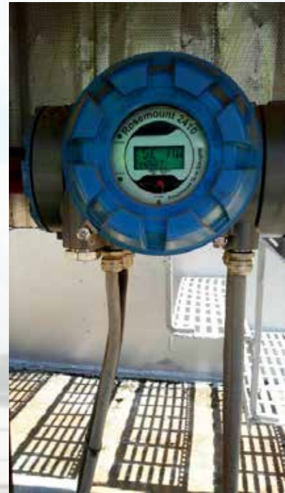
Tank Hub/Side monitor
