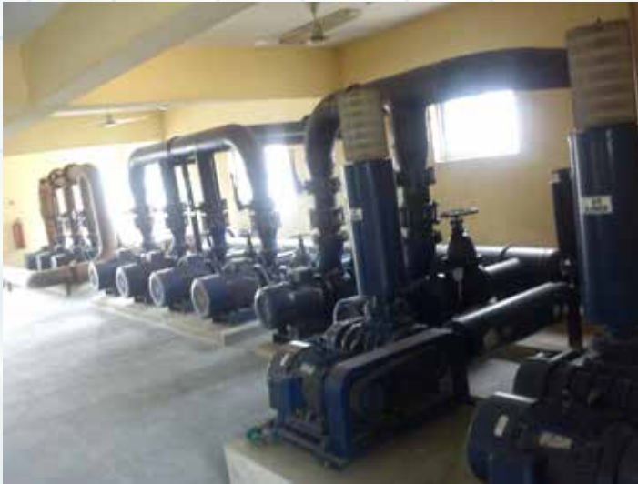
Booster and water transfer pumps installed in a water works.
